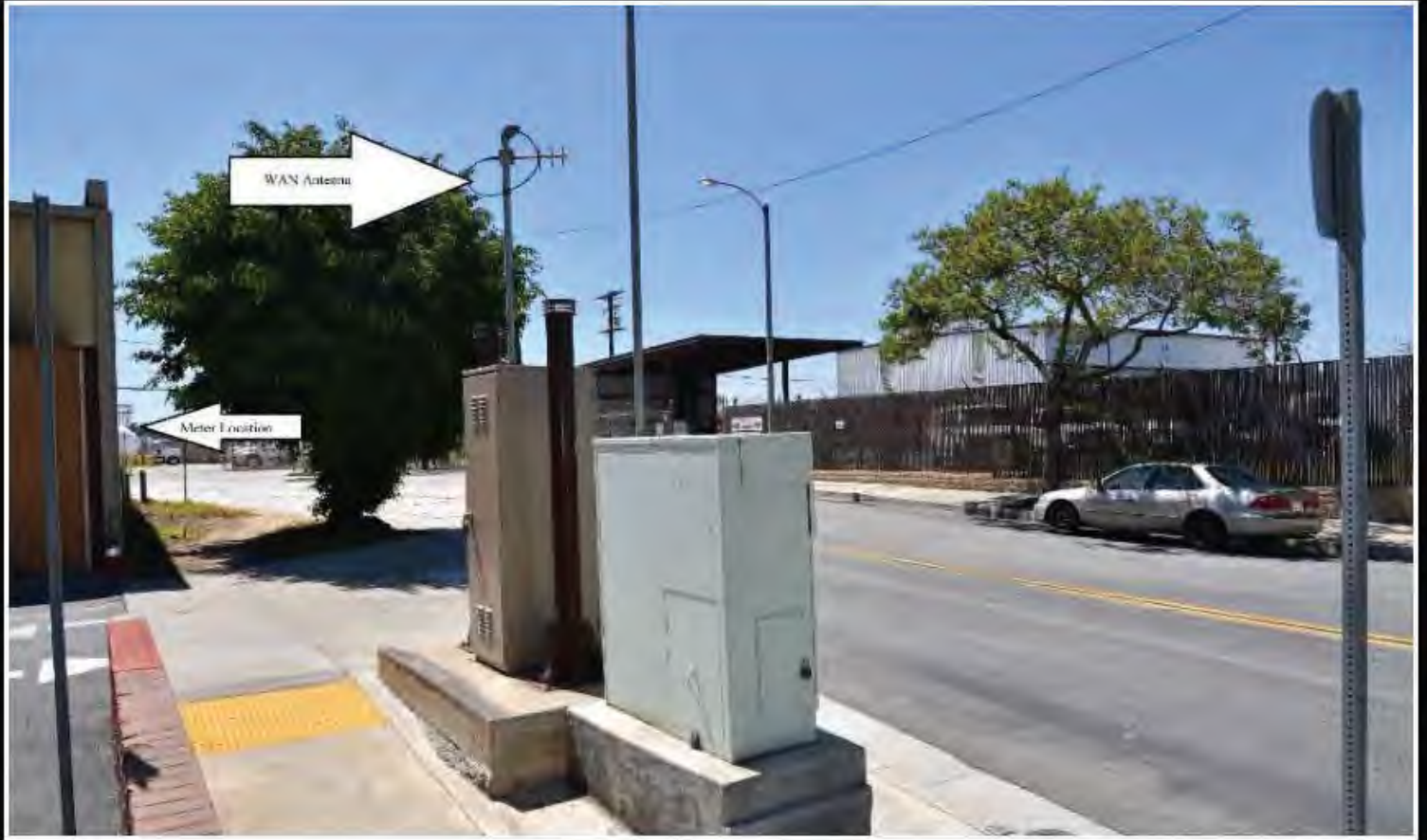
Sends Signals to WAN Antenna
